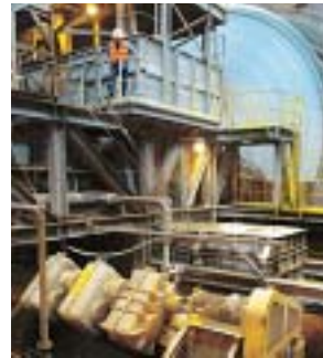
A SEMI-AUTOGENOUS GRINDING MILL in PT Freeport Indonesia's concentrating complex was a workhorse in 2003 – contributing to the 1.3 billion pounds of copper and 2.5 million ounces of gold produced at record low average unit net cash costs.
